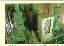
Main discharge pump of Zempukaji River intake facility
