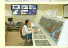
Control monitor and control board of Zempukaji River intake facility
