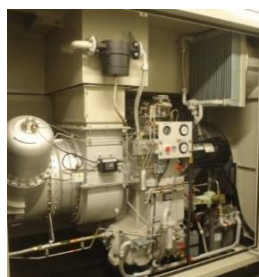
Figure 7. In-house Power Generation Facility
