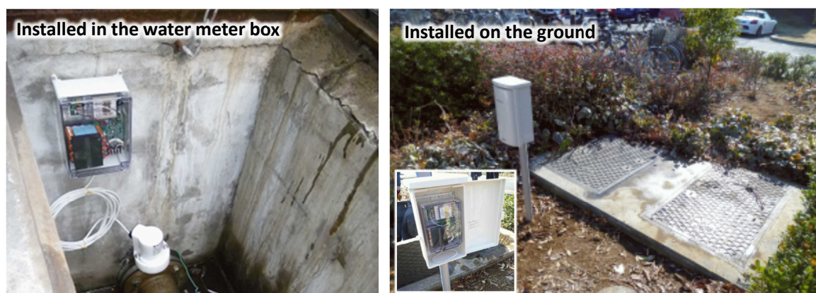
Figure 9 Installed data conversion/transmission apparatus
