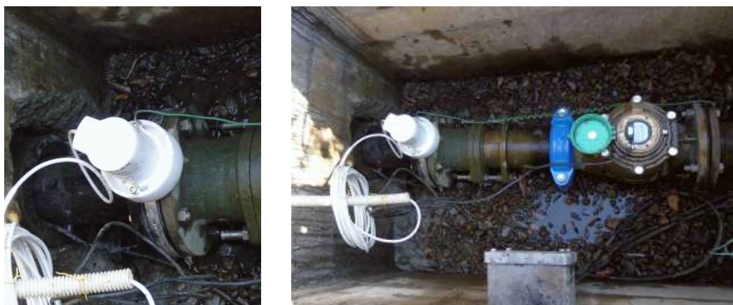
Figure 8 Installation of pressure sensor
