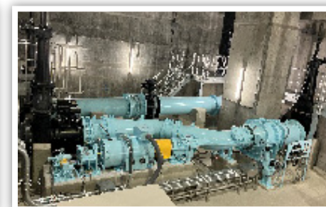
Small Hydropower Facilities (Kamikitazawa Water Supply Station)
