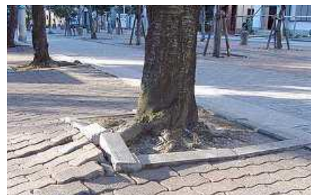
Uneven sidewalk due to rising tree roots
