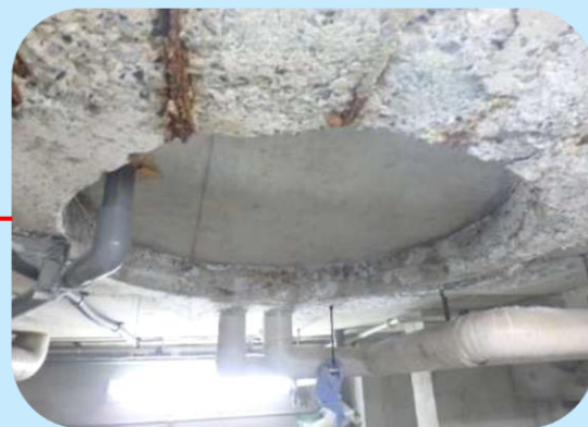
Corrosion of reinforced steel and deterioration of concrete
