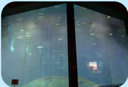
Cloudy acrylic and deterioration of glued parts
