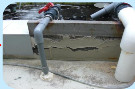
Deterioration of concrete (of the water tank)
