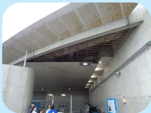
Corrosion of the ceiling bed
